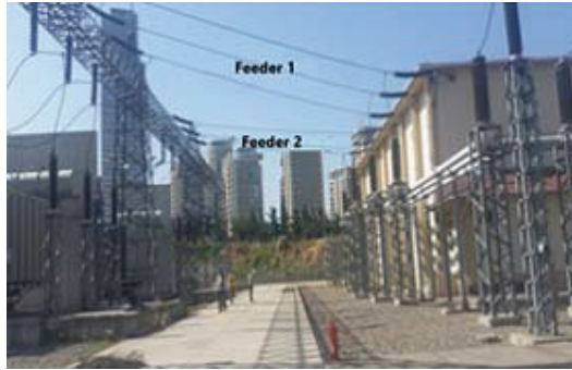
Figure 4: The 400/154 kV substation in field measurements
